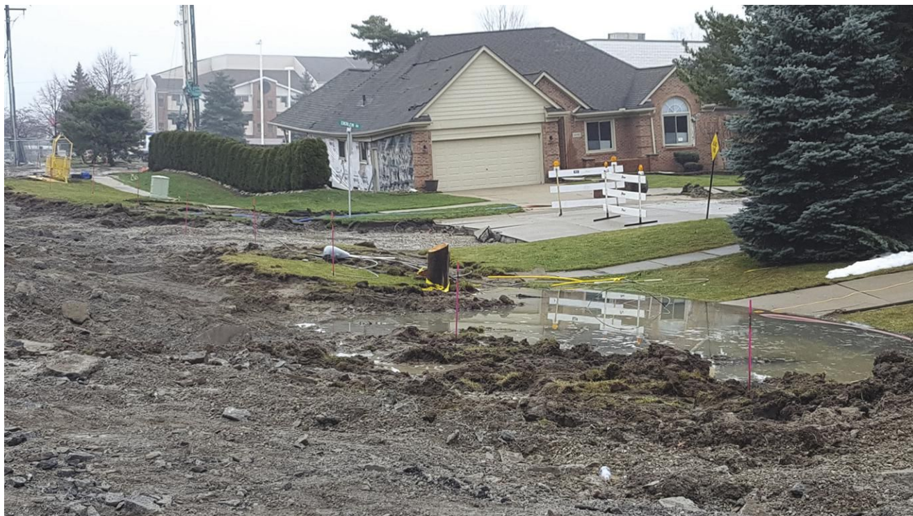
A sinkhole interrupted critical sewer flows and cut off access to a subdivision of 23 homes, where all residents were evacuated on Christmas Eve day, 2016.
