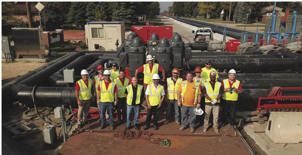
The critical nature of the project required personnel on site 24/7 from Christmas Eve until mid-October when substantial completion of the repairs was achieved.
