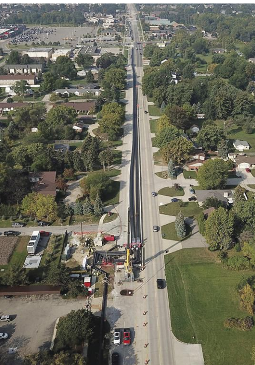
Repair of the damaged 11-ft-dia sewer interceptor involved over a mile of 48-in. and 54-in. piping and eight large vertical turbine trash pumps.
