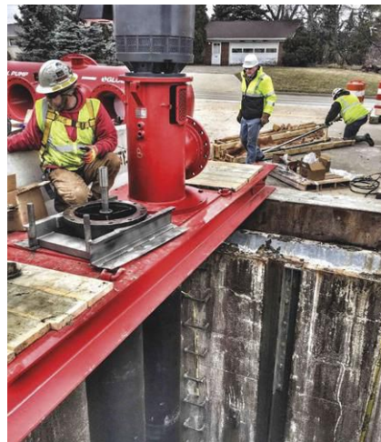
Mersino diligently constructed eight vertical turbine pumps suspended into the 60-ft-deep, 11-ft-dia interceptor pipe.
