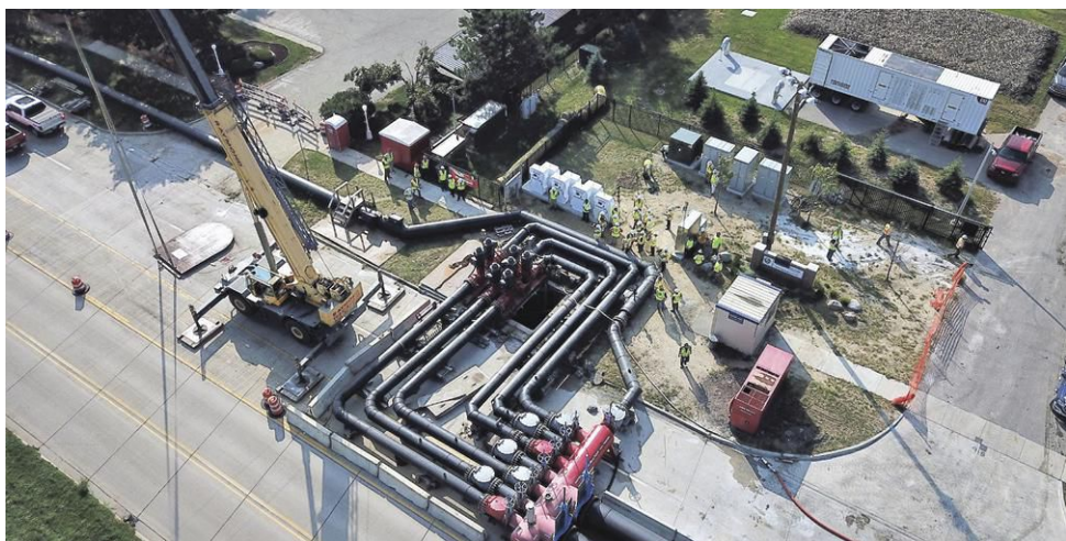
Featuring 1.25 miles of pipes, eight massive pumps, and high-tech communication and telemetry software, construction crews maintained normal interceptor flow, preventing raw sewage from being discharged into the Great Lakes.
